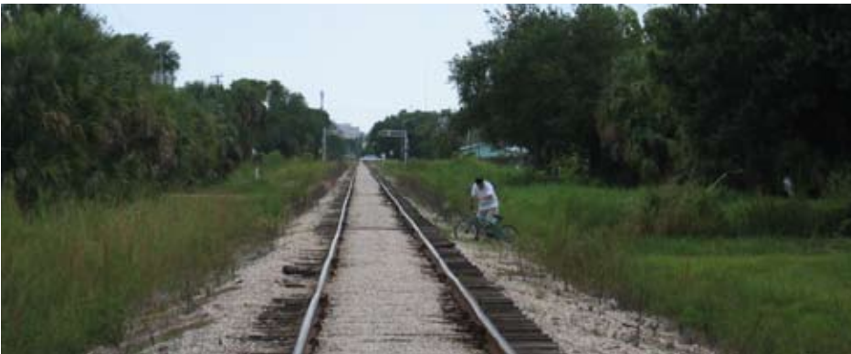
Figure 1.7: Poorly maintained rail lines and right-of-way.
