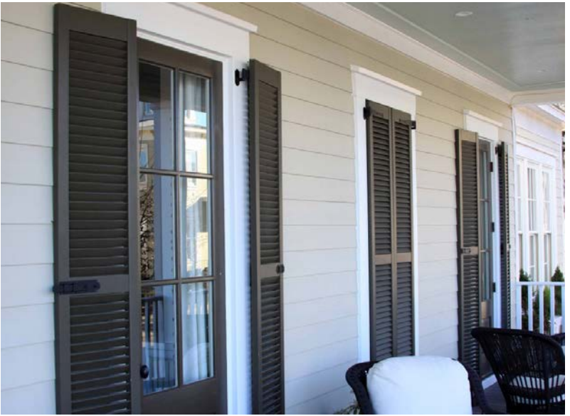
SHUTTERS. Shutters should be operable and sized to cover the opening they flank.
